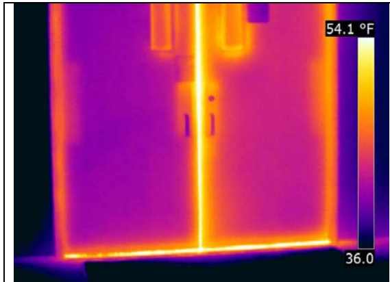
"HH 3-10" Energy loss around door
