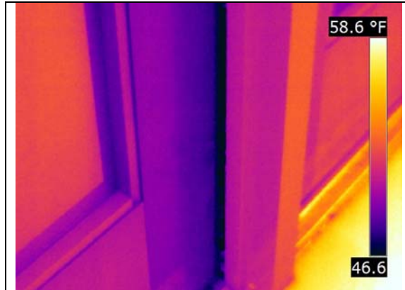
“HS 2-3” Energy loss around door
