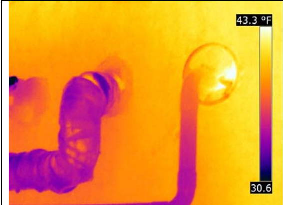
"B" Energy loss around penetration
