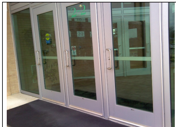
“HS 2-2” Recommend door seals
