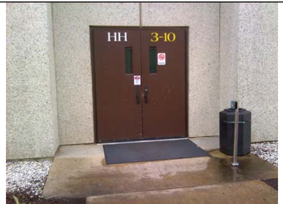
"HH 3-10" Recommend weather strip and door sweeps
