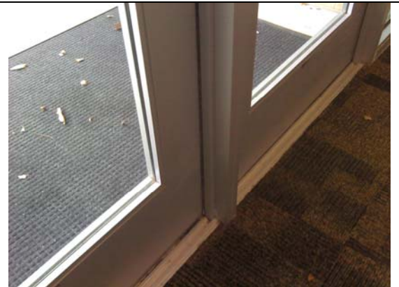
“HS 2-3” Recommend door seals
