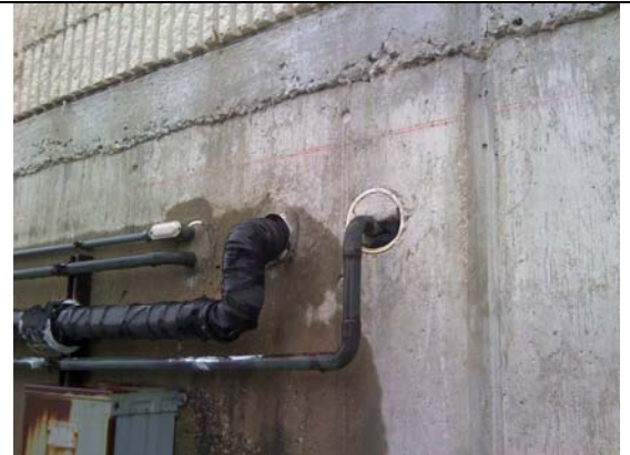
"B" Recommend sealant around penetration
